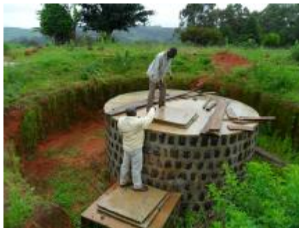
Edwin Visi our consultant engineer working with a villager on a storage tank.
